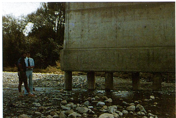
Figure 10.3: Degradation resulting from gravel extraction has left the pile cap high and dry – Ohau River Bridge.
