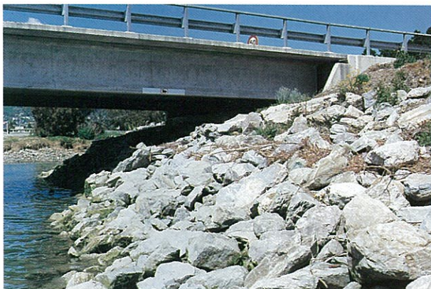
Figure 10.8: Moonshine Bridge – Hutt River illustrates the use of riprap to protect an abutment.
