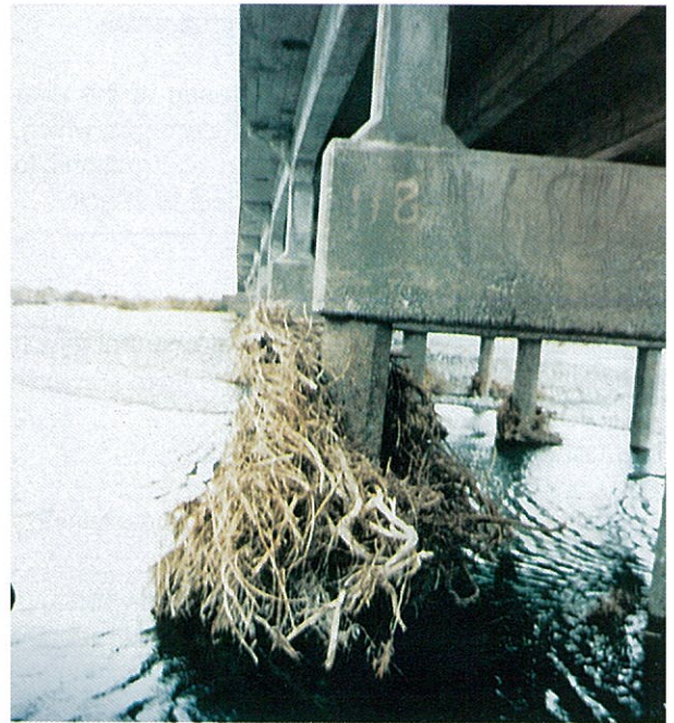
Figure 10.6: Accumulation of debris against bridge piers.
