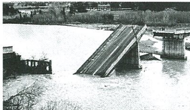
Figure 10.4: The Bulls Bridge over the Rangitikei River failed as a consequence of local scour around the pier foundations in 1973.
