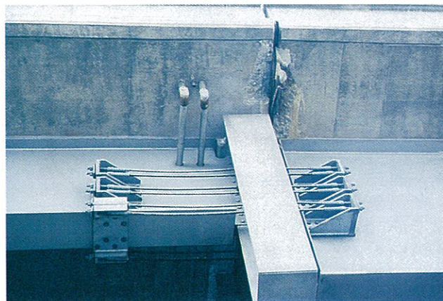
Figure 11.1: Spalling damage at expansion joint.
