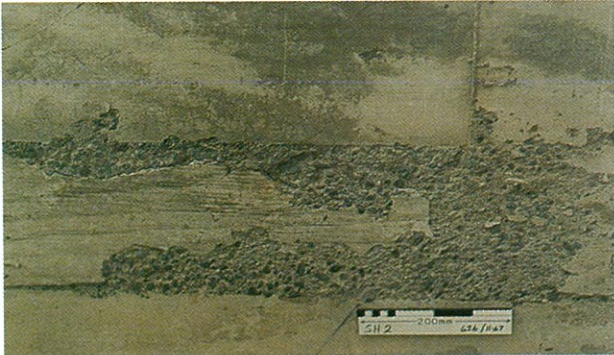
Figure 3.4: Surface mortar can be removed by frost
