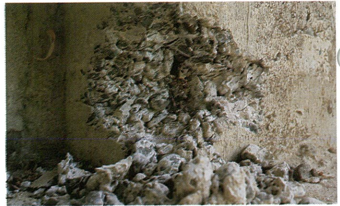
Figure 3.5: Honeycombed concrete and associated reinforcement corrosion
