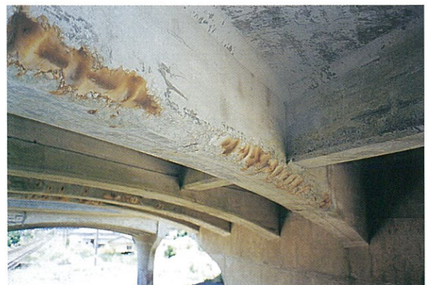
Figure 3.8: Continuing reinforcement corrosion where repaired with epoxy mortar
