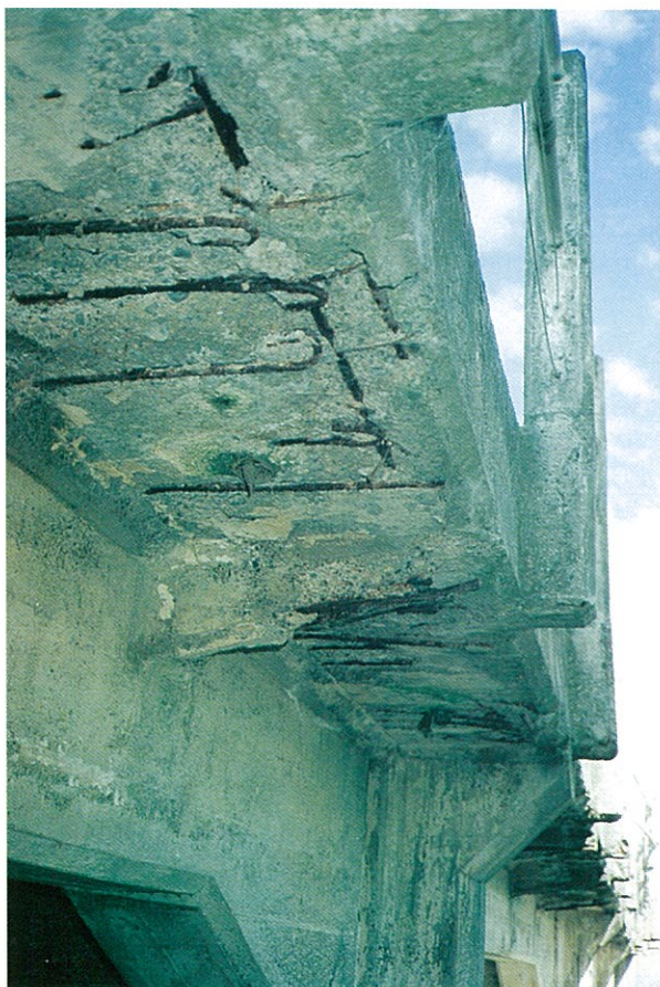
Figure 3.2: Spalling due to extensive reinforcement corrosion on a deck soffit.
