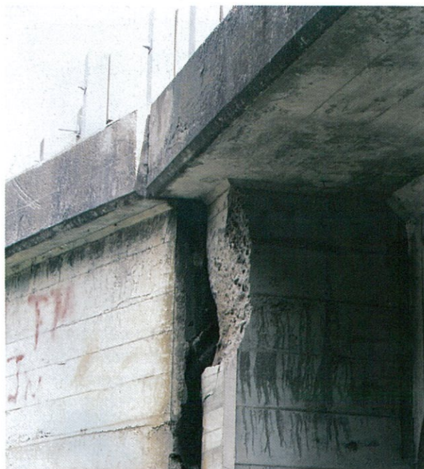
Figure 3.3: Spall caused by seismic movement.
