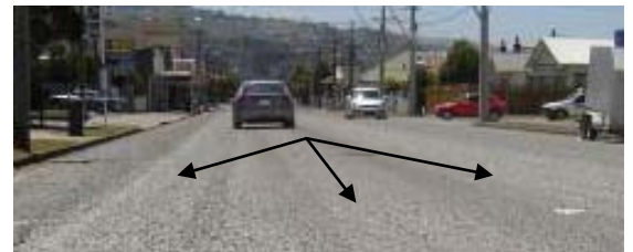
Too much loose chip on seal surface and on road shoulder
