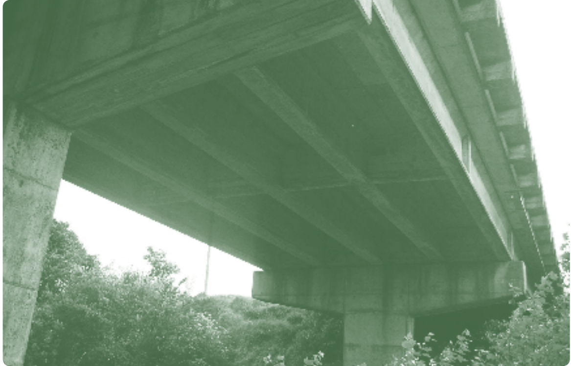
A typical concrete bridge superstructure. Corrosion of reinforcing or pre-stressing steel is one of the main durability problems affecting concrete pier caps, beams and decks.
