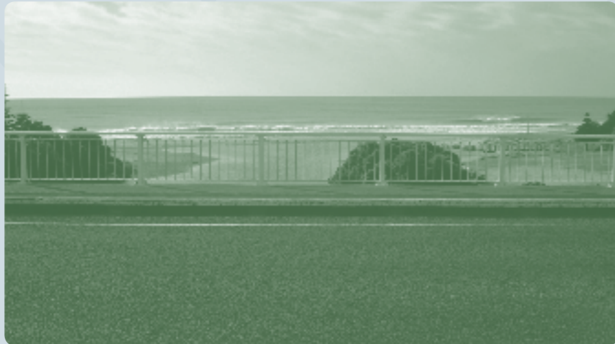
The bridges most likely to benefit from treating concrete surfaces to prevent or slow the corrosion of reinforcing and pre-stressing steel are those exposed to splash or spray from seawater, such as this bridge near a surf beach.
