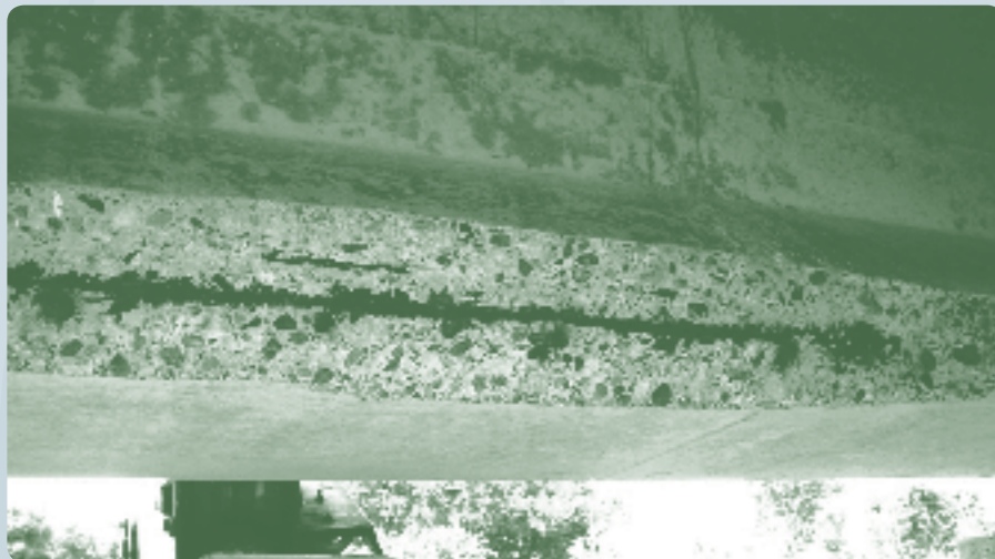
Close-up of rusty strand and rebar.
