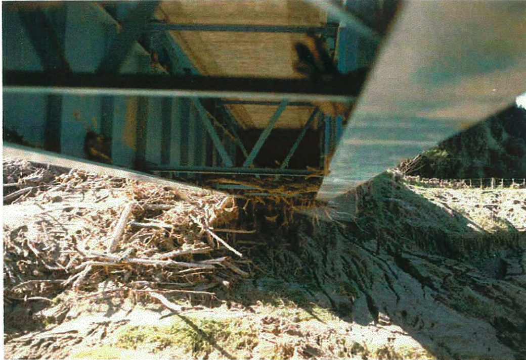
Figure B9. Debris accumulations on the bridge superstructure.
