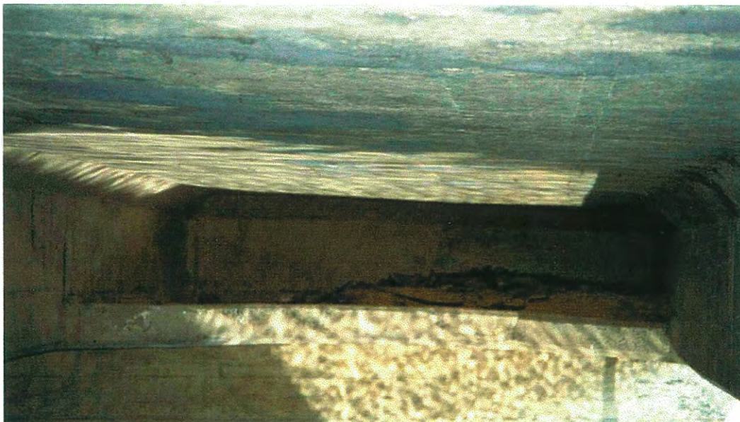
Figure B10. Sediment deposits on the bridge superstructure (on top of a pier and immediately below the bridge deck).
