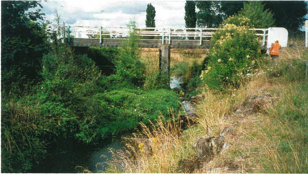
Figure B7. Bridge waterway significantly blocked by vegetation; note also the fencing across the waterway that could potentially aid debris blockage of the channel; flow is away from the viewer.
