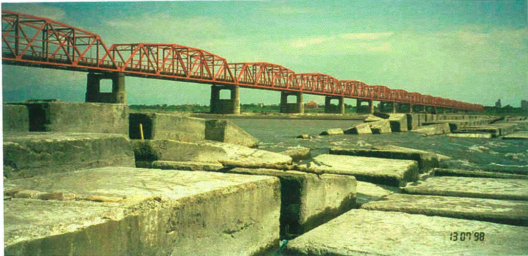
Figure B5. Undermining and lowering of a weir designed to control degradation at the upstream bridge; flow is to the right.
