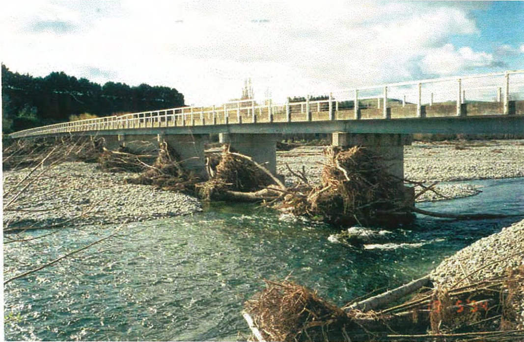
Figure B21. Debris accumulations on bridge foundations; flow is to the right.
