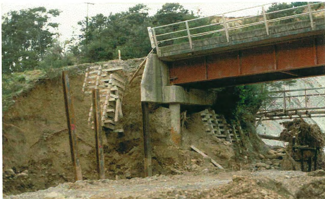
Figure B16. Toe erosion and fill movement providing evidence of undermining of a spill-through abutment; equivalent evidence would be apparent for the undermining of a bridge approach. Note the associated damage to the existing countermeasures evident in the photo.
