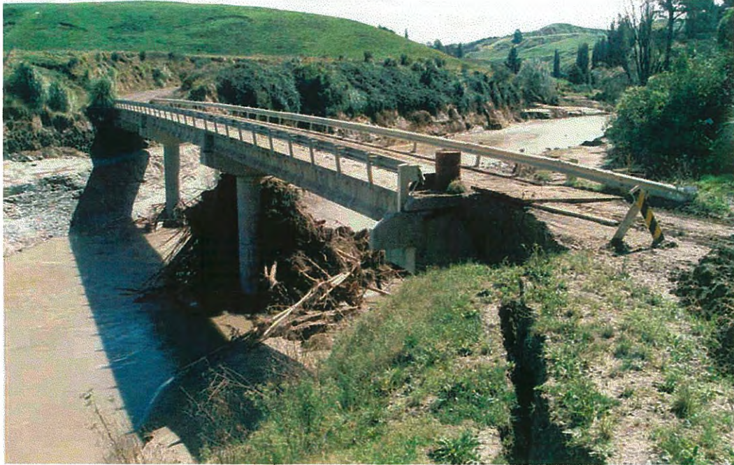
Figure B11. Ongoing bank erosion/ failure at the bridge site, as indicated by a significant tension crack along the top of the near bank and the vegetation-free region of notable thickness along the base of the far bank. A significant debris accumulation has formed against the central pier. Flow is to the left.
