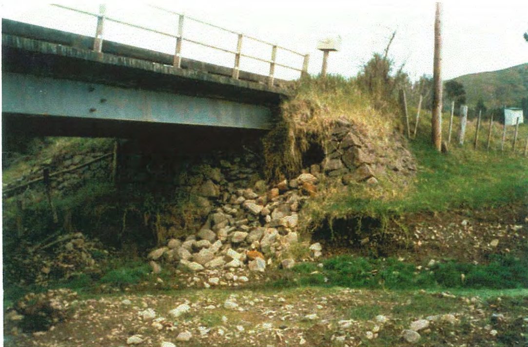
Figure B17. Toe erosion and fill movement providing evidence of undermining of a spill-through abutment; equivalent evidence would be apparent for the undermining of a bridge approach. Note the associated damage to the existing countermeasures evident in the photo.
