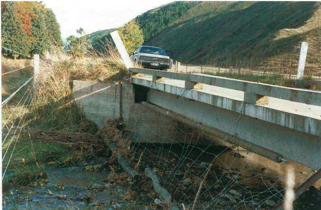
Figure B8. Bridge waterway significantly blocked by fencing that could potentially aid debris blockage of the channel; flow is to the left.
