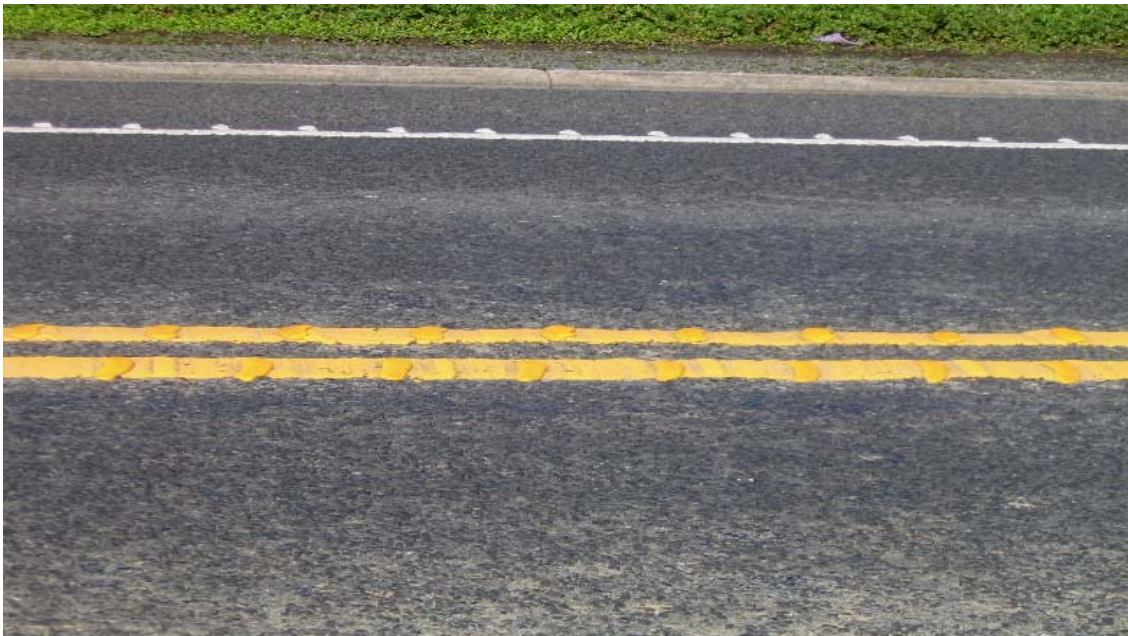
Figure 4.1 New ATP ribs installed on top of an existing ATP centre-line resulting in inconsistent rib profile and spacing which fails to meet specifications
