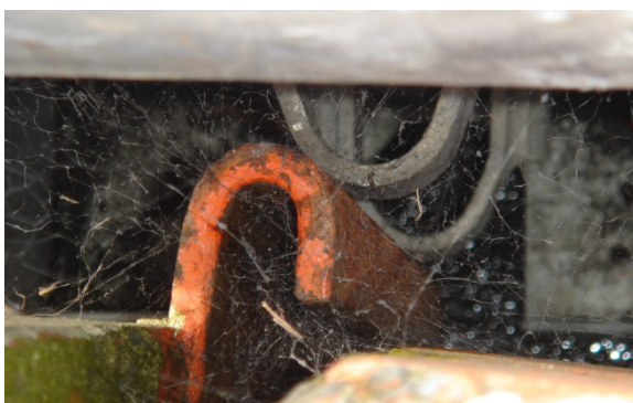
Figure 2: Incorrect pairing (JJ Hooks on left)
