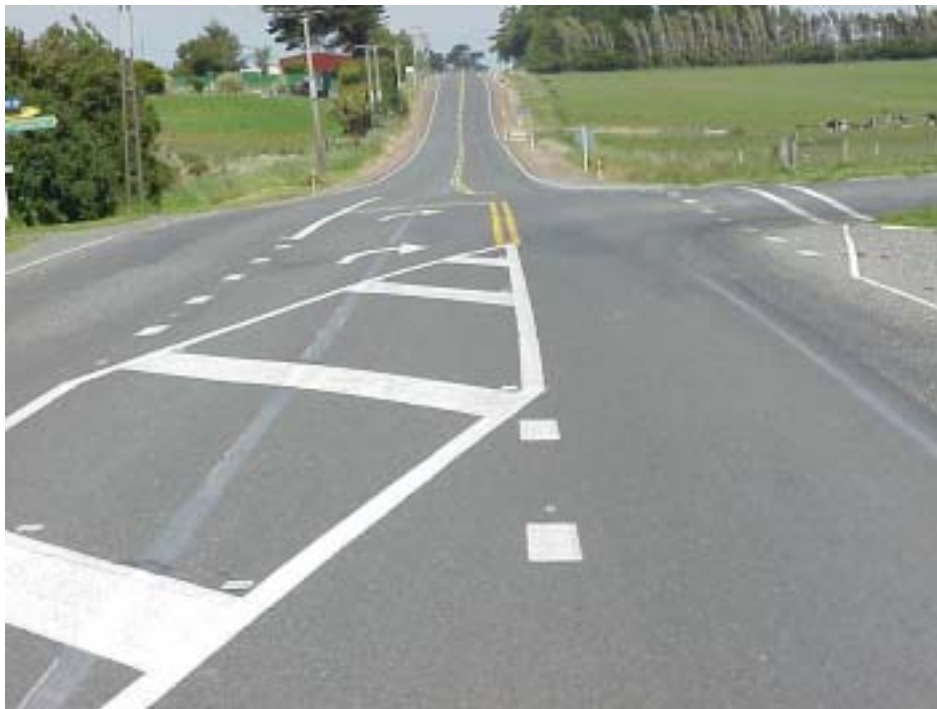
Unsafe delineation from 'blacked out' unwanted centre and edge lines. Glass bead was clearly evident on the blacked out markings. Tests showed these lines had higher reflectivity than the new white lines and would therefore be more visible at night (reflectivity readings of 111 and 64 on the blacked out lines, compared with 58 to 80 on the new white lines).
