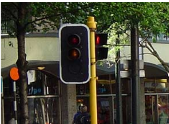
Figure 9 Non-complying two-aspect display (green missing)
