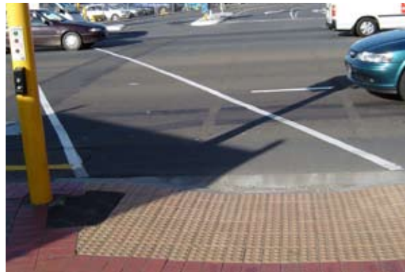
Figure 16 Visually impaired pedestrians are directed away from the crosswalk by the warning paver layout. Tactile pavers should be laid at the same angle as the crosswalk
